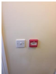
Upstairs Alarm Activation Button
