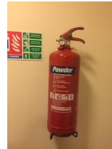
Kitchen Upstairs Fire Extinguisher
