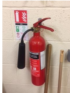
Kitchen Downstairs Fire Extinguisher
