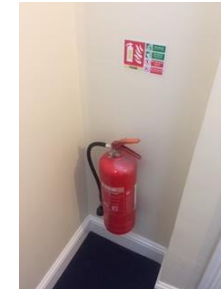
Top of Stairs 1 st Floor Fire Extinguisher
