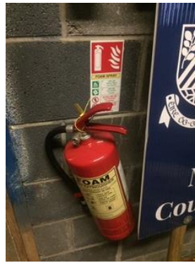
Kit Room Fire Extinguisher
