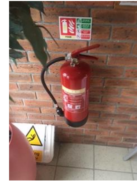
Left of Main Club Door Fire Extinguisher
