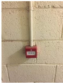
Main Hall Alarm Activation Button
